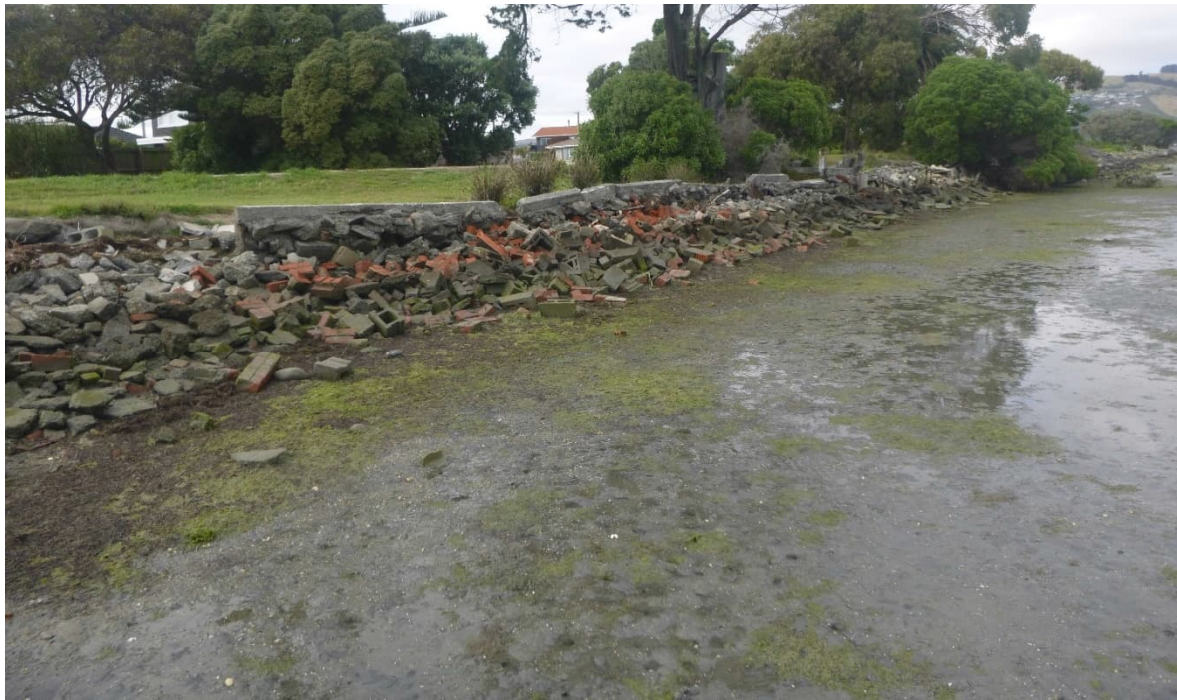
Figure 7-44. Facing southeast, showing the sea wall made up of cement blocks, bricks, and parts of concrete walls.
