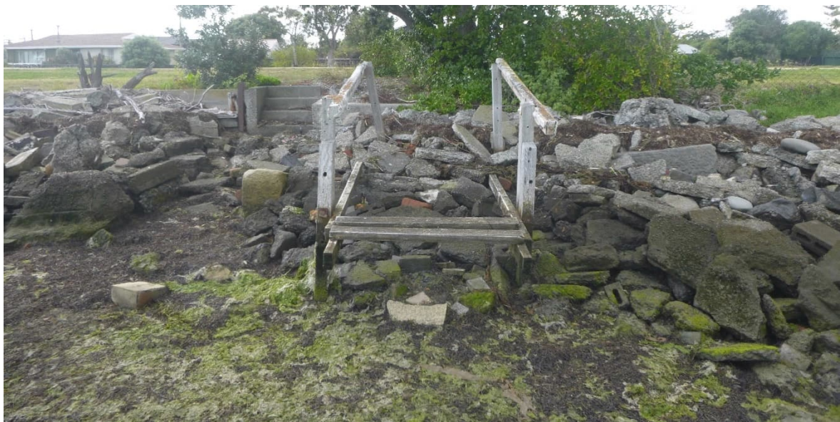
Figure 7-45. Facing east, showing derelict wooden structures at the estuary edge.
