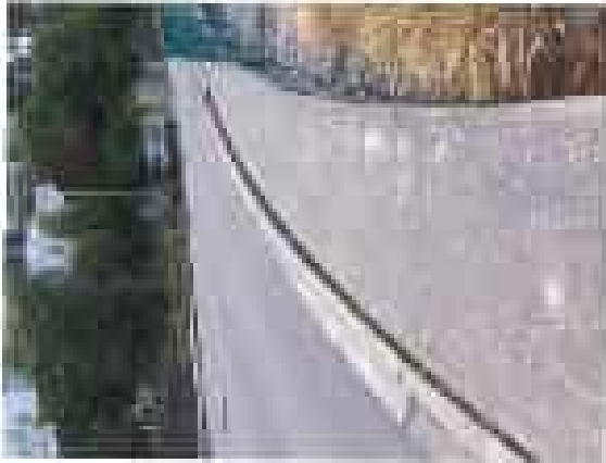
Kerb elevated above footpath
