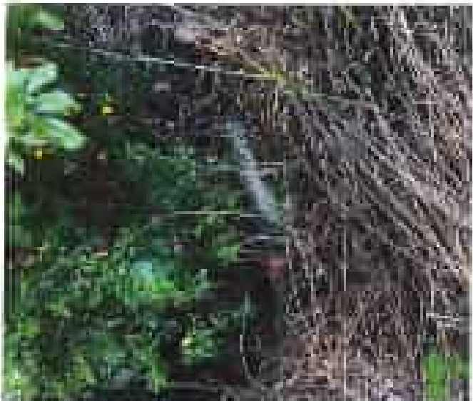
Over grown main storm water sump
