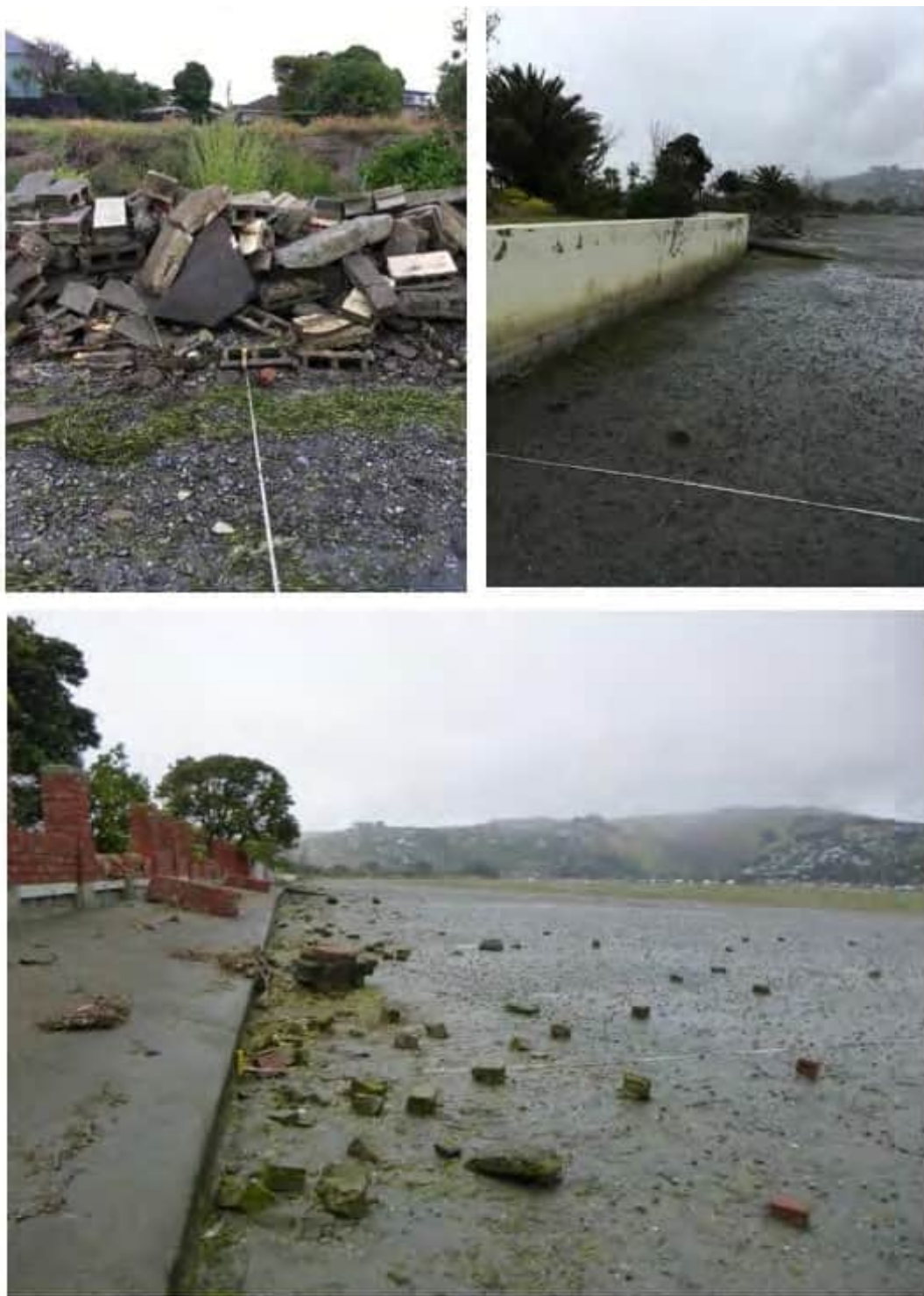
Figure 11. Examples of artificial structures along the estuary edge, with debris littering the seabed.
