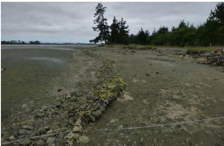
Figure 9. Erosion resulting in the formation of new areas of seabed behind the reno mattresses used to protect the former shoreline at South New Brighton Park.
