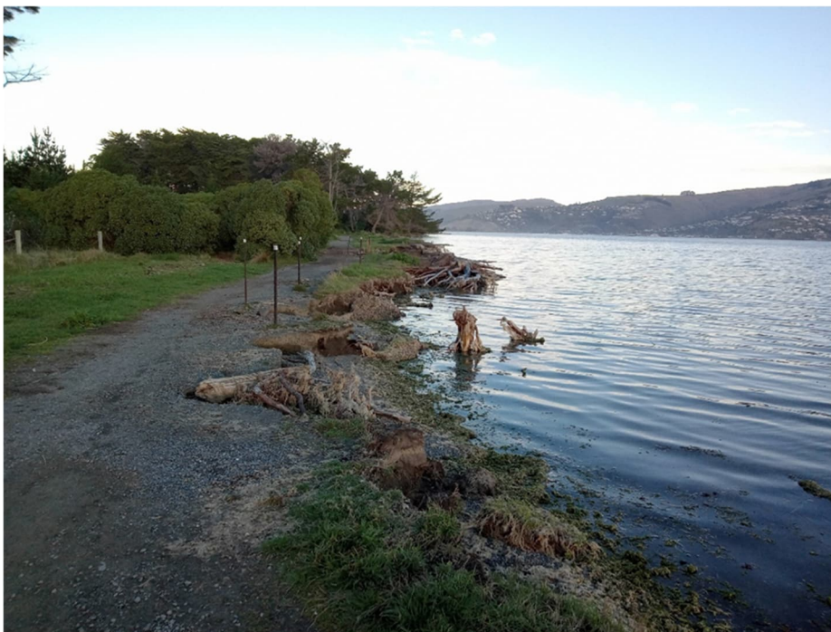
Figure 25 Submerged reno mattresses in a spring tide with walkway through the park eroding (June, 2021)
