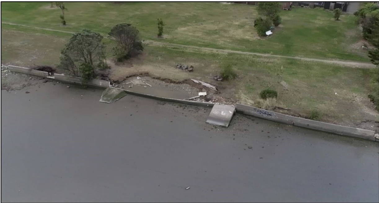
Figure 4 Erosion behind low lying failed structure in Southshore estuary edge area (Jacobs, 2019)
