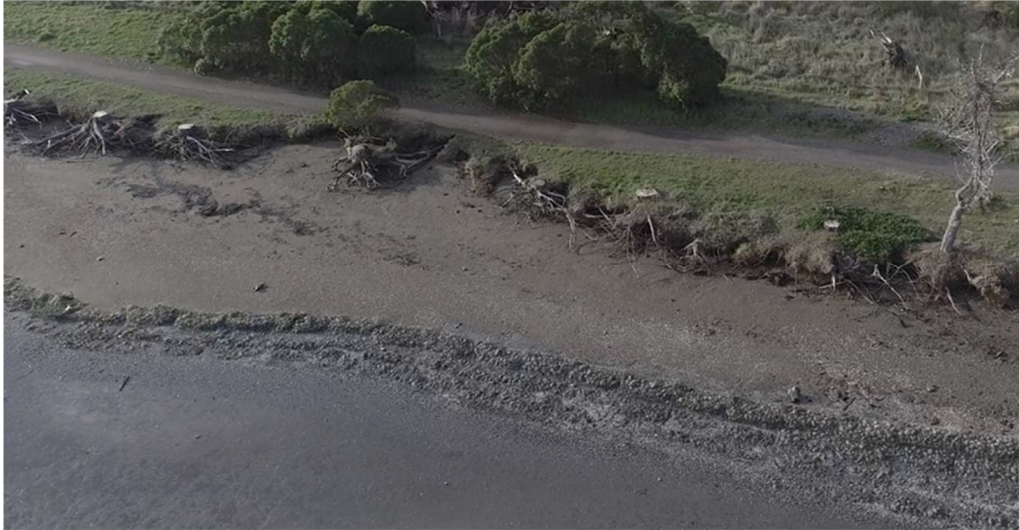
Figure 24 Erosion behind low lying reno mattress structures in SNBP (ECan, 2019)
