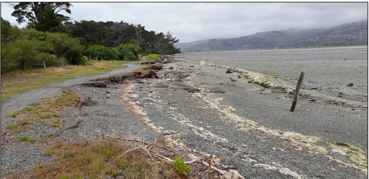
Figure 7 Another example of erosion behind slumped reno mattresses in South New Brighton Park impacting the existing coastal path in the park (photo taken January, 2022)
