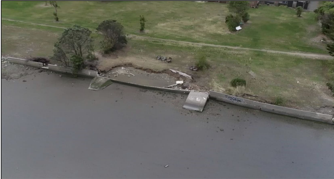
Figure 26 Erosion behind low lying structures in Southshore (2019)
