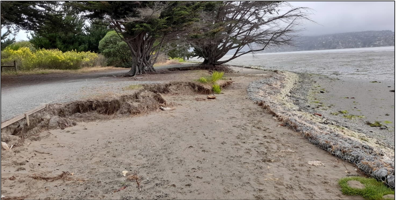
Figure 6 Example of erosion behind slumped reno mattresses in South New Brighton Park impacting the existing coastal path in the park (photo taken January, 2022)
