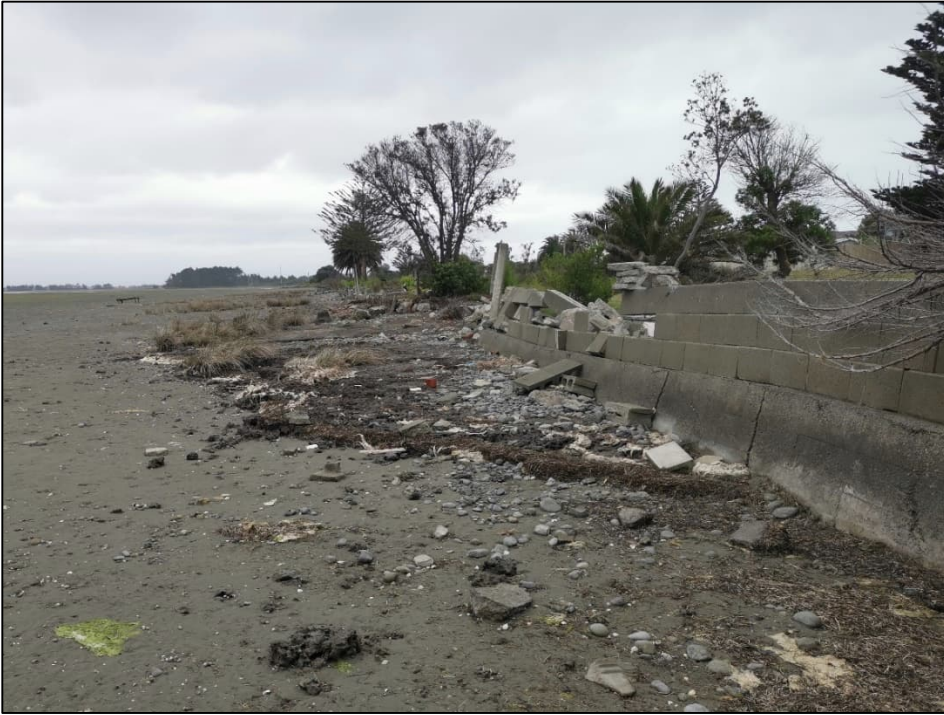
Figure 2 Example of failed erosion protection structure along red zoned land in Southshore (photo taken January 2022)
