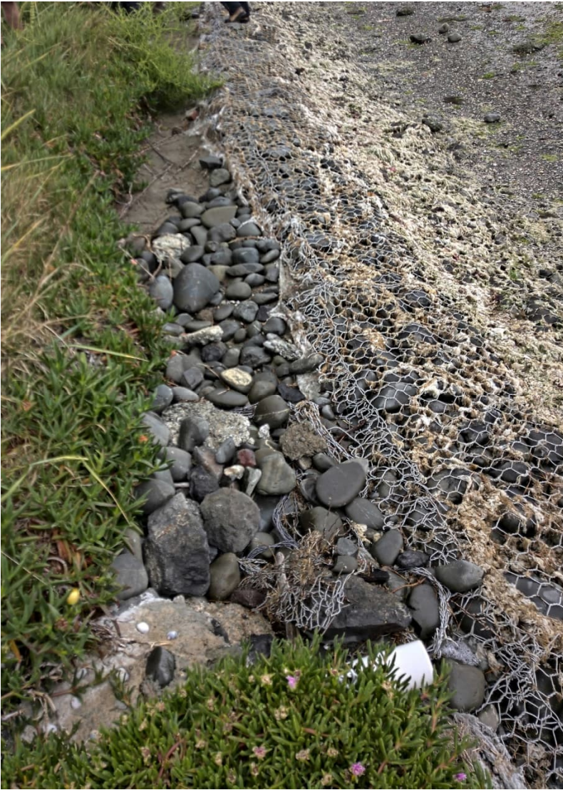
Figure 5 Example of failed gabion baskets/reno mattress in South New Brighton Park showing areas of broken wires and erosion occurring (photo taken January, 2022)
