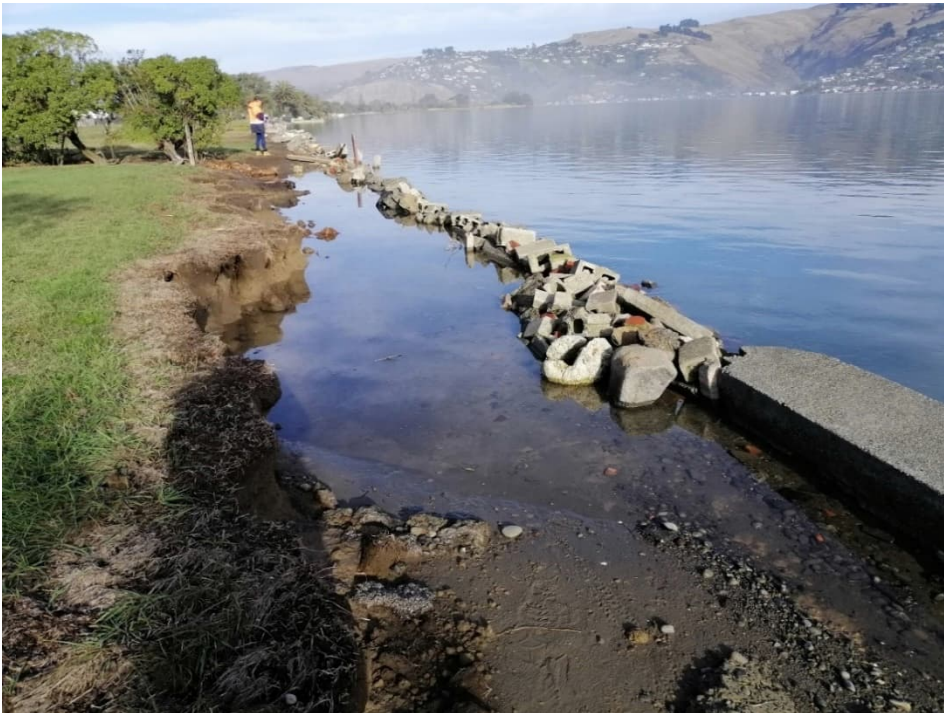
Figure 3 Low lying structure in Southshore overtopped in a high tide with erosion scarp behind (photo taken 2022)
