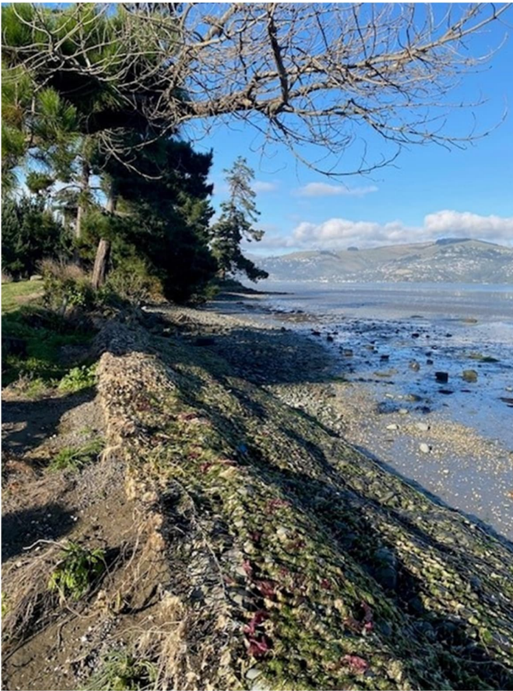
Figure 30 Erosion at SNBP (2022)
