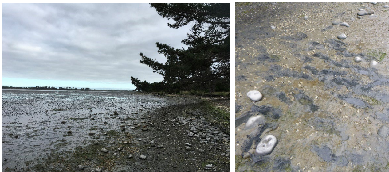
Figure 3. Cobble material from the damaged reno mattresses scattered across the mudflat habitat at South New Brighton Park.
