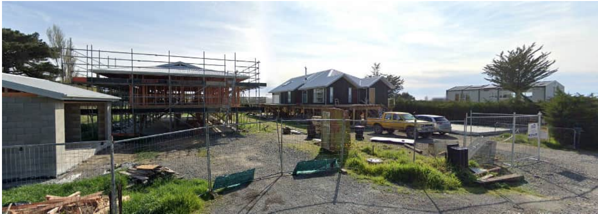
Figure 13: Earlham Street Residents Have Built Homes with Finished Floor Levels Greater Than 2m Above Ground To Deal With The Regular Flooding
