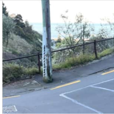
Power pole on footway mid stretch road bend. Beat up by number of times it has been scraped by vehicles cutting the corner and going on footway. NB: Area is already yellow lined.
