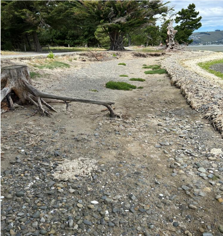
Figure 2: Photograph of existing consented reno mattress shoreline protection, with erosion behind, along the South New Brighton Park edge. (Source: Application Documents).
