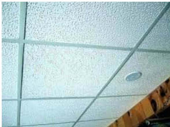
Textured ceiling tiles containing asbestos
