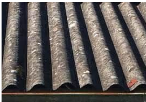
Super 6 roofing corrugations containing asbestos
