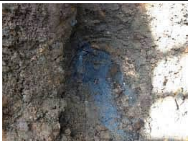
Discoloured soil and water in the base of an excavation.
