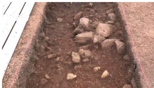
Unexpected building rubble in an excavation.
