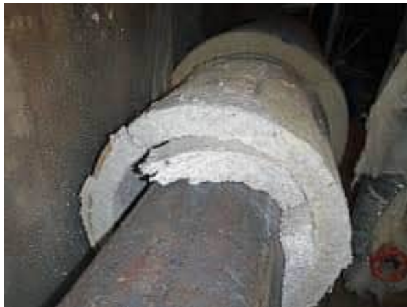
Asbestos insulated pipework
